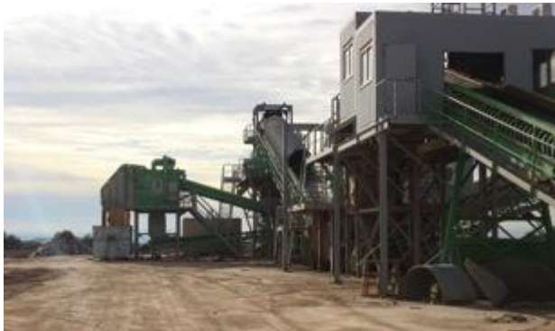
Figure II-16 Stationary recycling plant in south Madrid
