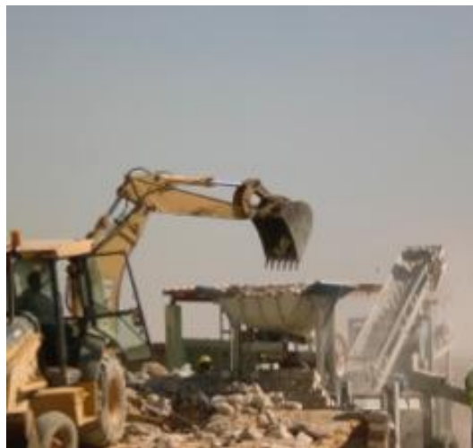
Figure VI-2 Crusher 50 TPH (case study)
